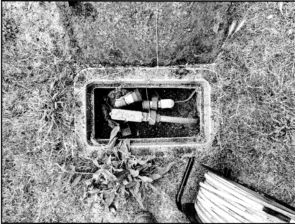
Photo 3: View of Observation Well OW-2B.
