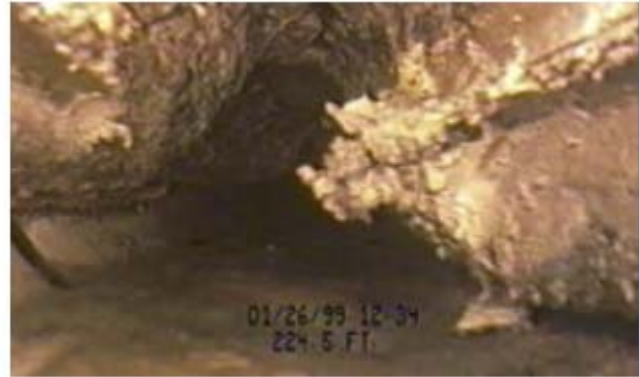
Grease clogged sewer
