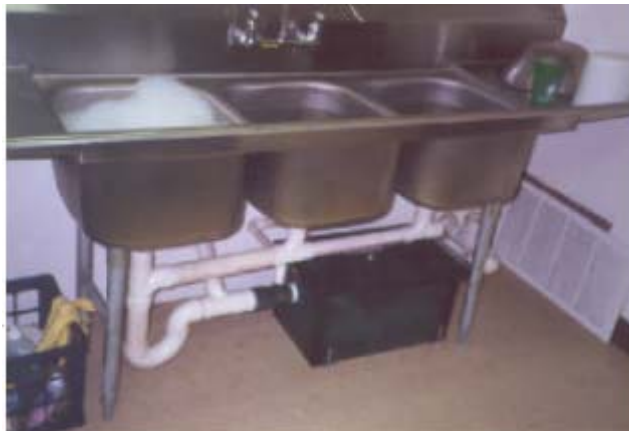
Grease traps must be cleaned frequently
